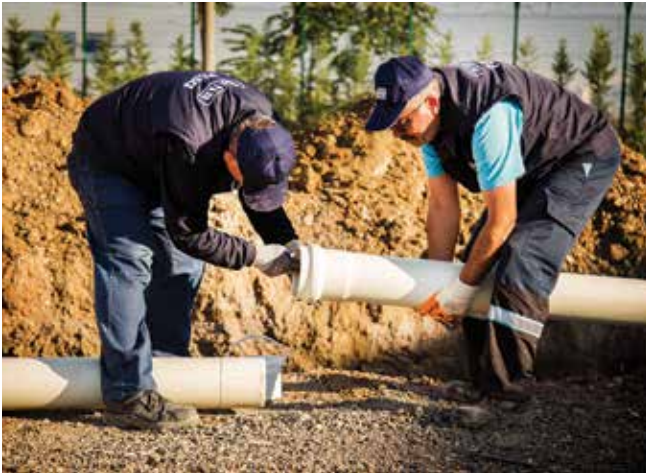
Clean the pipe and spigot parts with high care, before connecting the pipes to each other.
